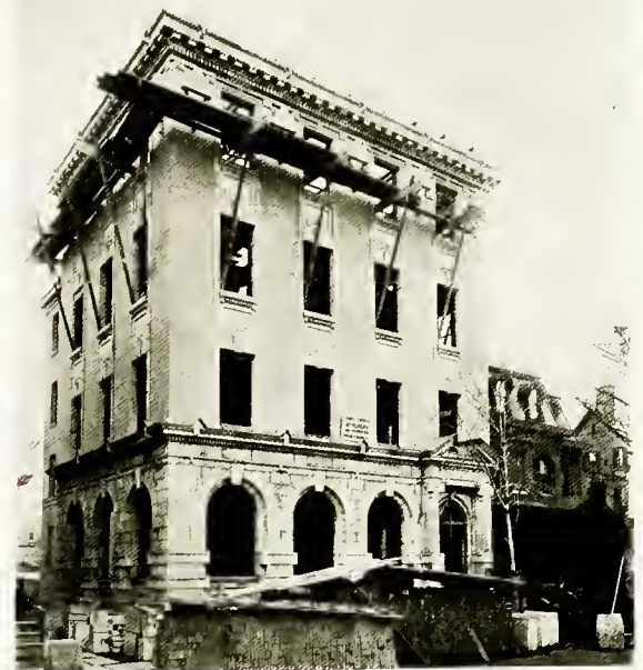
Spring Brook Water Supply Co. Office Building N. Franklin St. (Under Construction)
